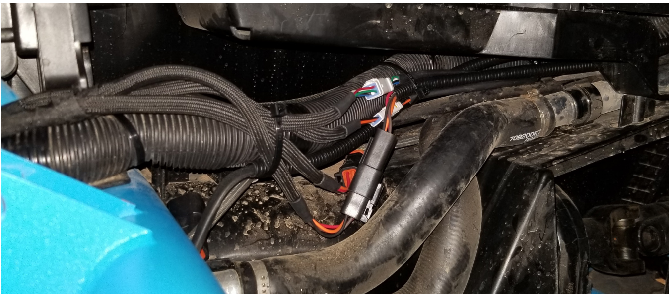
Figure 14b: Shows a secured portion of the main harness towards the front of the center console.
